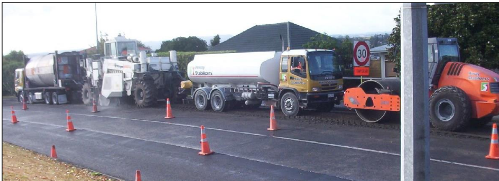
Figure 16: FBS in urban setting with an existing central concrete strip that was retained
