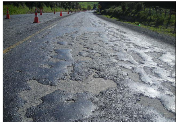
Figure 12: October '07 major surfacing failure
