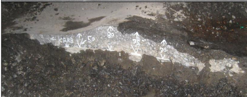
Figure 10: Trenching by the Client confirmed relief was entirely in membrane / asphalt surfacing with a level FBR surface
